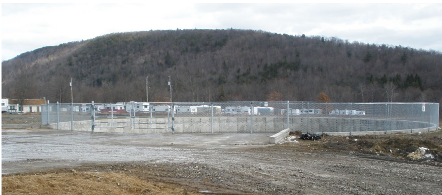
Installed total collection system for silage leachate
